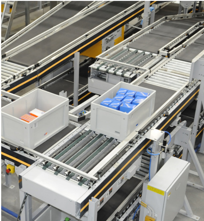
Plastic totes are conveyed and transferred using motor driven rollers
